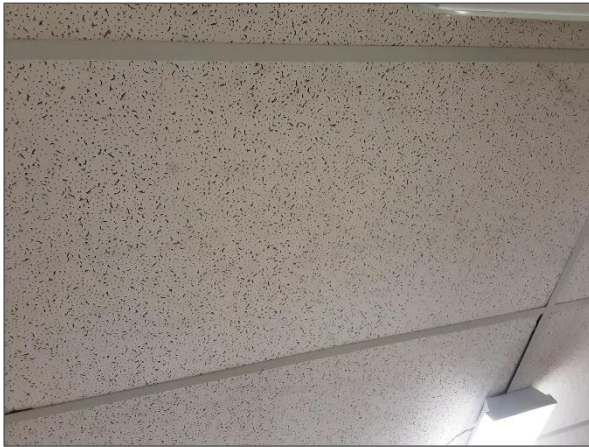
Non-asbestos lay-in ceiling tiles with small pinholes, small fissures.
