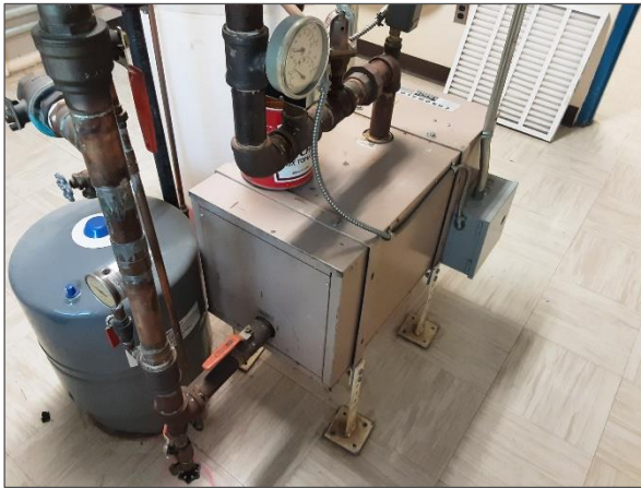
Furnace insulated with non-asbestos fibreglass.
