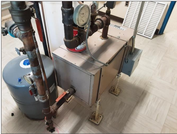
Furnace insulated with non-asbestos fibreglass.
