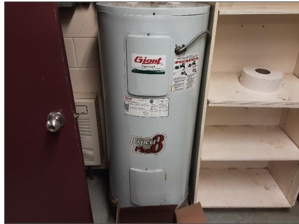
Hot water tank insulated with non-asbestos fibreglass.
