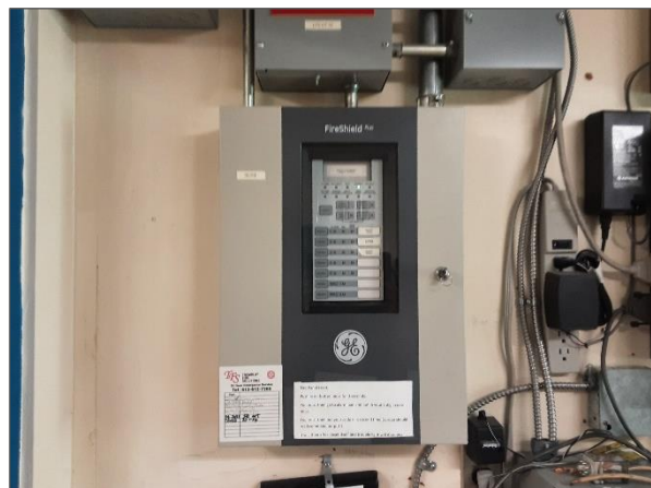
Lead-containing batteries in fire alarm control panel.
