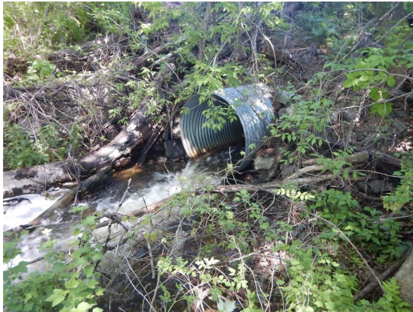
Photo 4: Perched Culvert Downstream of Tracks (May 18, 2022)
