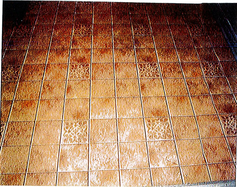
Photo 1: Location of samples S1, S2 and S3 (vinyl sheet flooring in basement) for asbestos testing. This material did not contain asbestos.
