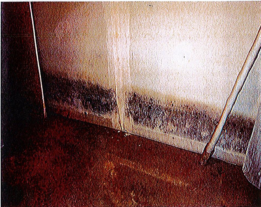
Photo 10: Possible black mould found on the drywall in the basement.
