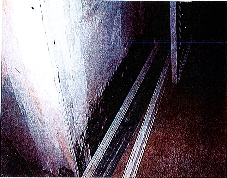
Photo 11: Possible black mould found on the drywall in the basement.
