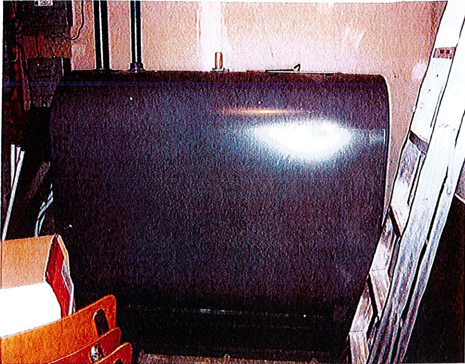
Photo 9: Heating oil tank located in the basement. Possible benzene present.
