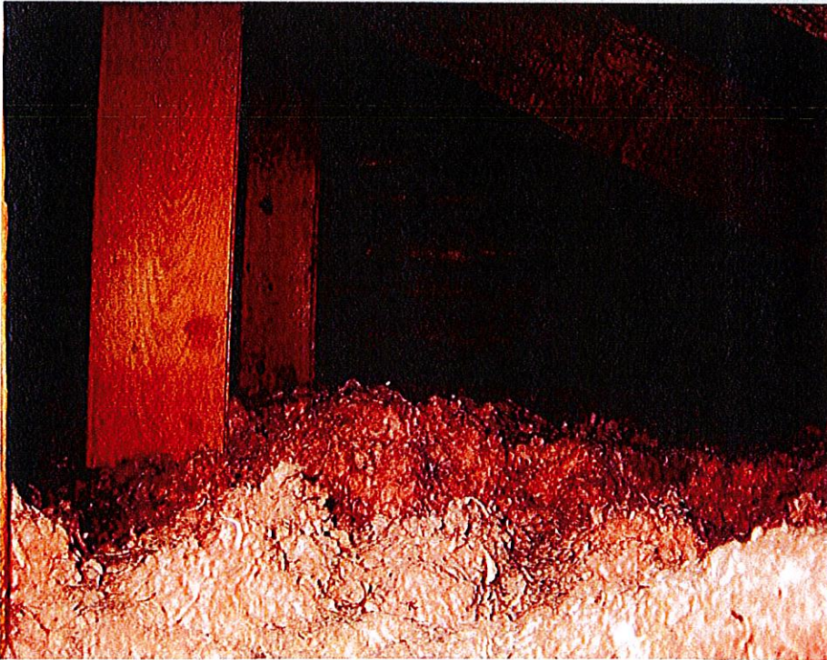
Photo 12: Blown in, loose fiberglass insulation found in the attic space.
